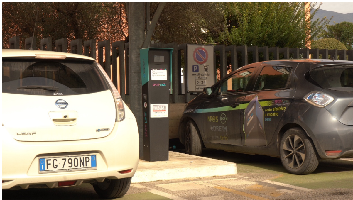
Figure 9: Emotion's electric vehicle charging stations
